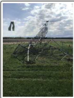
Downed Power Lines North of 84th and Havelock in Lincoln NWS Damage Survey
